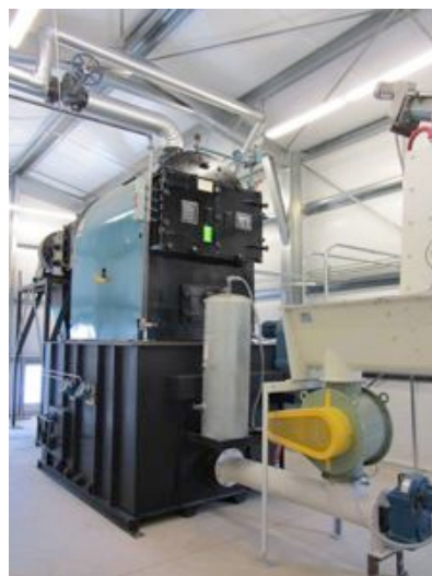
Figure 17. Biomass Combustion Systems Pellet Boiler (photo by Wisewood Inc)
