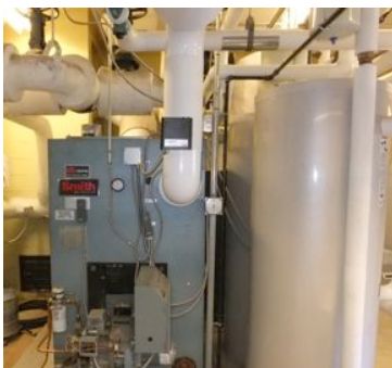
Figure 7. Heating Oil Backup System
