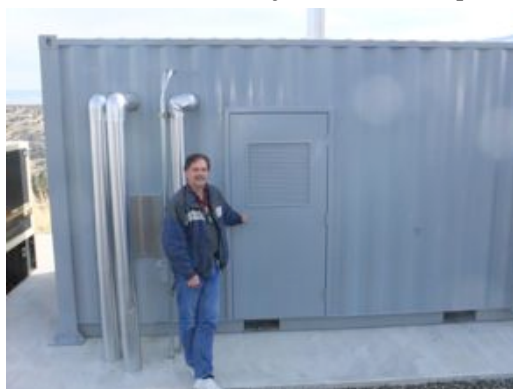
Figure 11. Patrick Bentz, Airport Manager, Next to the Pellet Boiler Container
