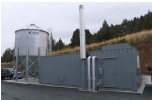
Figure 8. Pellet Silo and Biomass Housing Unit
