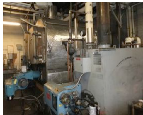
Figure 9. Heating Oil Boiler
