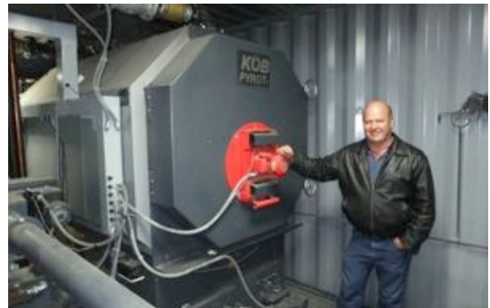
Figure 7. Steve Hill, Director of Facilities Services, Next to the Pellet Boiler
