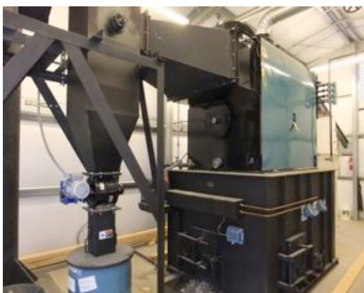
Figure 4. Rear of the Hurst Pellet Unit
