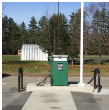
Figure 8. Diesel Fueling Station
