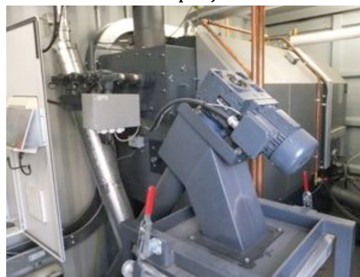
Figure 13. Side View of the Pellet Unit
