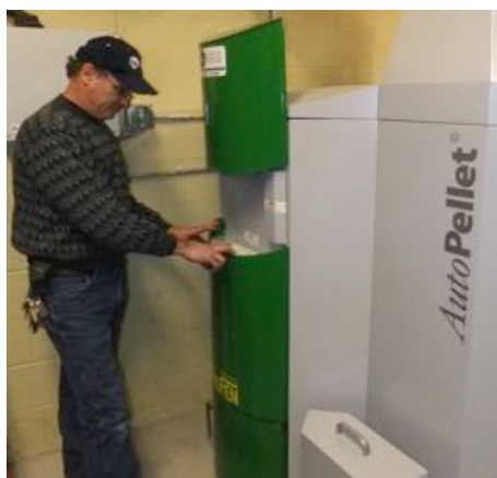
Figure 31. Operating Pellet Unit
